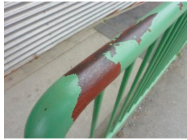
Handrail requiring repainting
